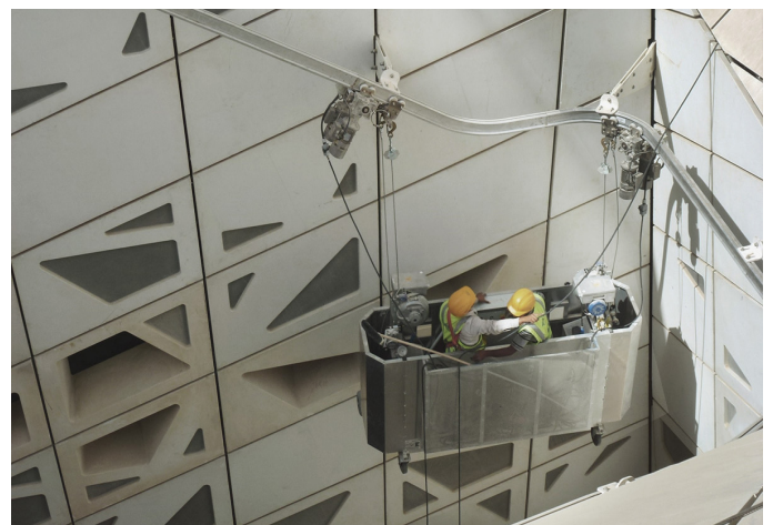
Cradle suspended from SafeAccess rail.
