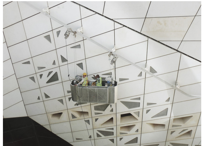
Maintenance of courtyards: SafeAccess monorail for cradle suspension.
