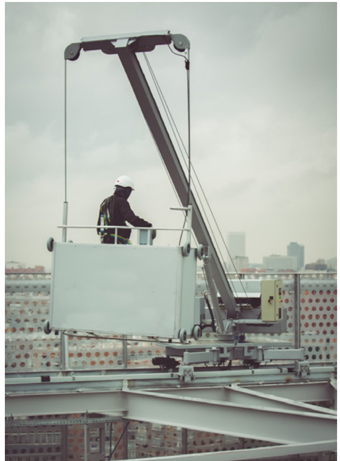
BMU FBA 1 installed in Spain. The rails are fixed to an upper structure behind a 3m high parapet. The machine has a jib luffing, in order to pass the cradle over the parapet.
