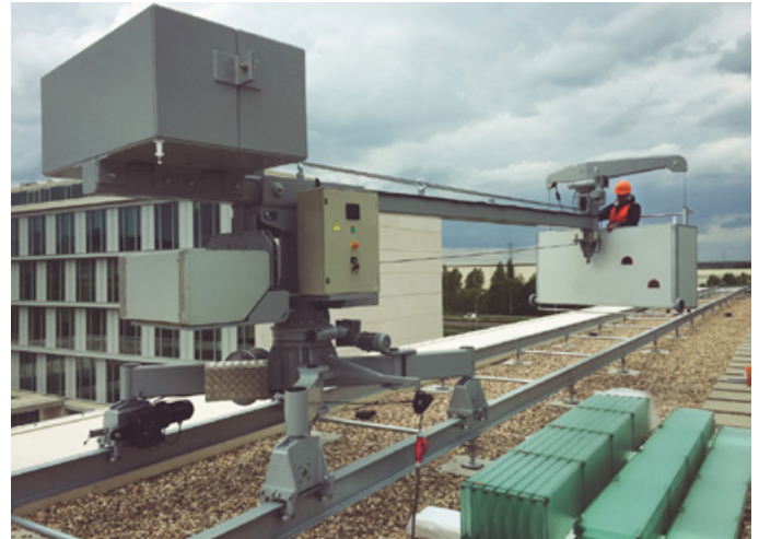
BMU FBA 1 installed in Luxembourg. Depending on the reactions that appear on the rails, these can be only supported, without fixings on the roof
