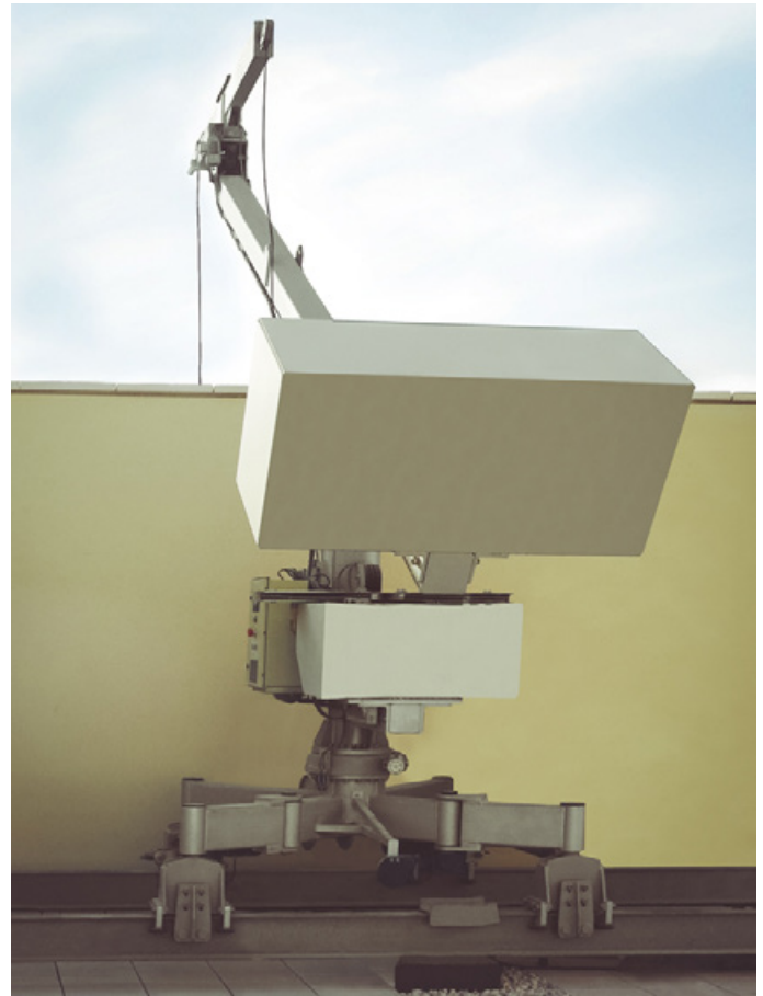
FBA 1 with jib luffing, in order to pass the cradle over the high parapet. Installed in Doha, Qatar.
