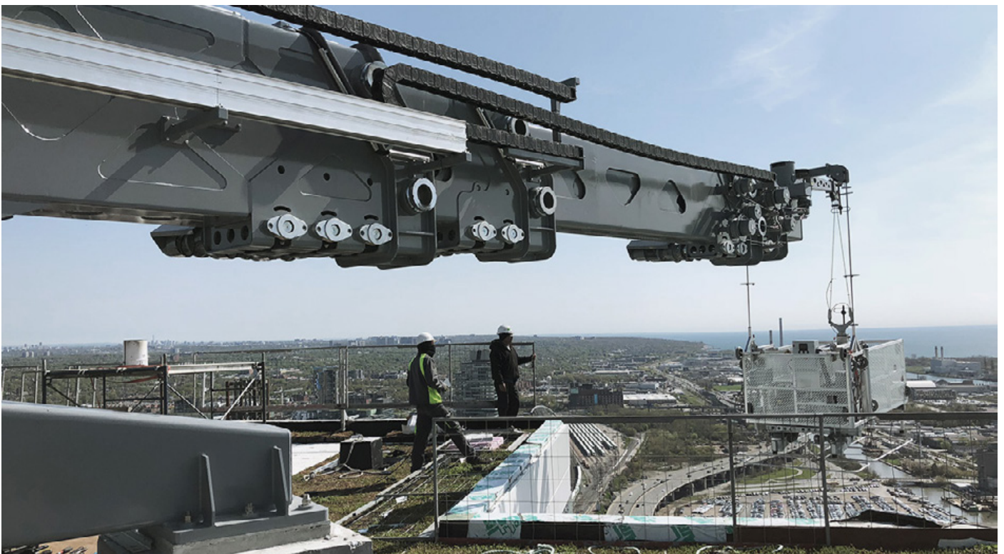
User operating the BMU through remote control from the building's terrace.
