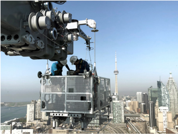
The 3-module cradle suspended from telescopic arm towards the city of Toronto.
