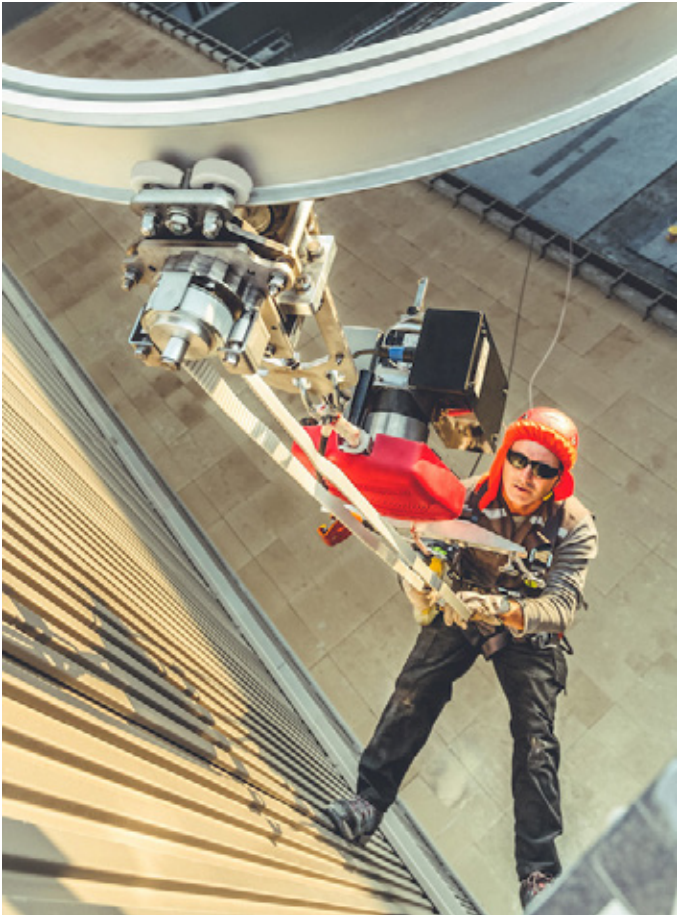
SafeAccess Monorail with RopeClimber which can be removed after use.
