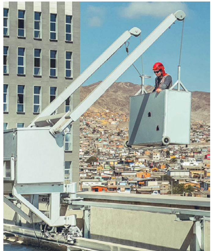
BMU type FBA 2 fixed on a rail-track attached to the inner parapet.
