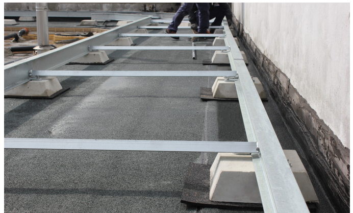
Installation of the rail track. This one has to be a freely laid track without any penetration on the roof in order not to damage the water proofing.
