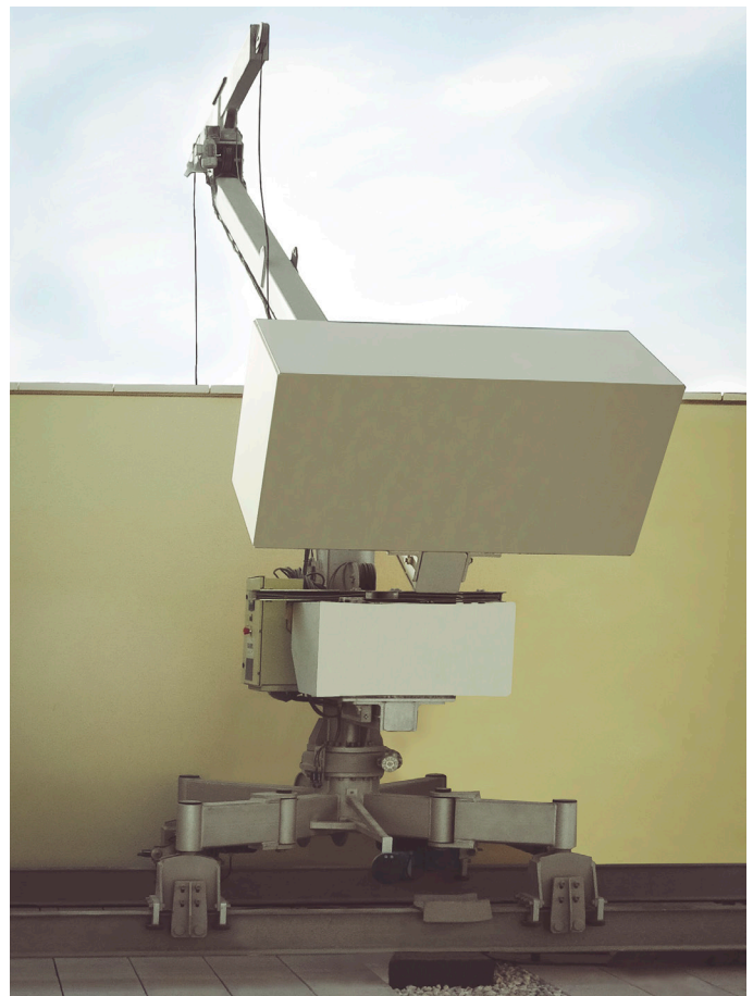
FBA 1 with jib luffing, in order to pass the cradle over the high parapet. Installed in Doha, Qatar.
