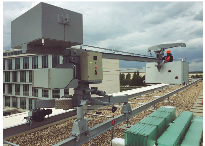
BMU FBA 1 installed in Luxembourg. Depending on the reactions that appear on the rails, these can be only supported, without fixings on the roof deck structure.
